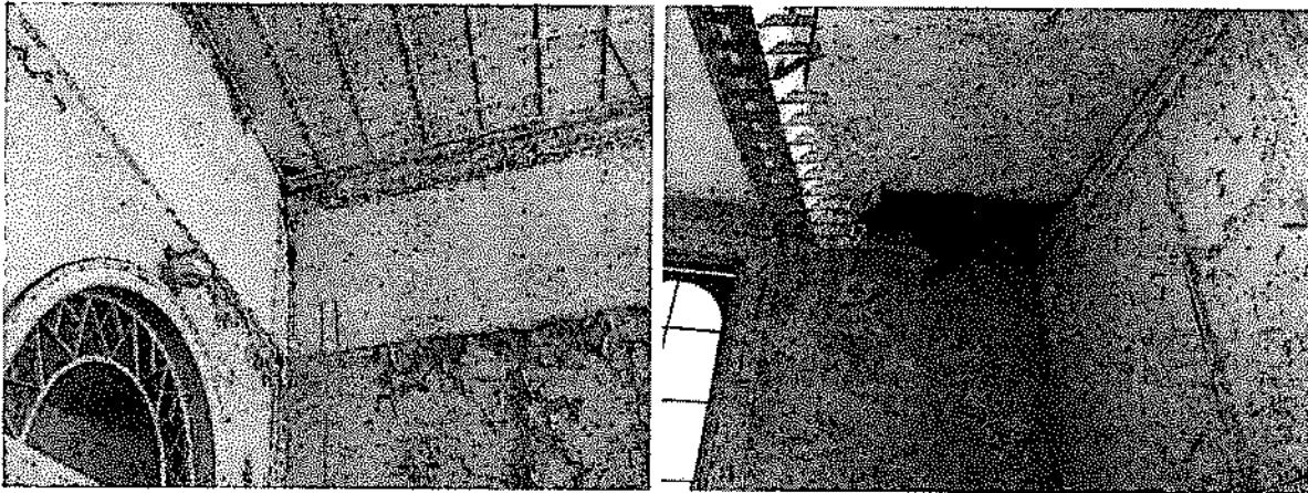
Water damage Date taken - 7/23/14 by Greg Zehr
